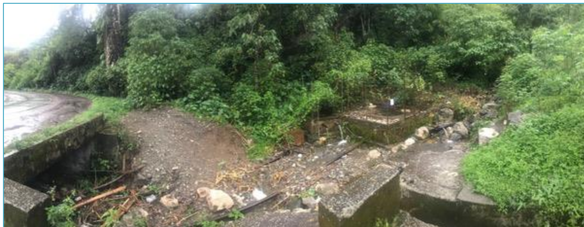
Plate 3- Erluli 1 Spring with existing Intake structure, BPT and pipelines
