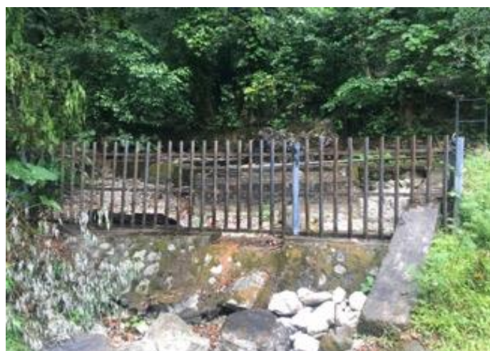
Plate 5- Darelau Spring with existing Intake structure and BPT
