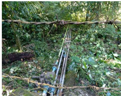
East view of SMASA & JICA Distribution Network System - Kotalala spring
